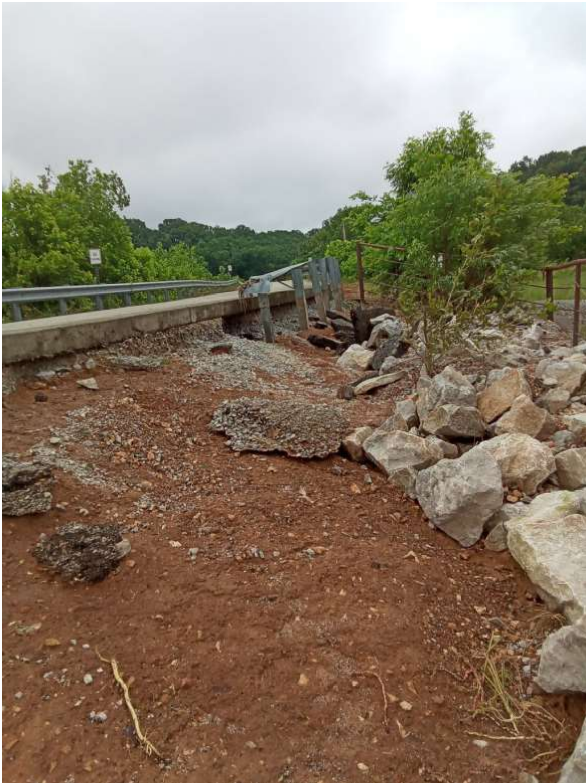
Emergency Procurement #2025-2 Road Damage Picture 1
