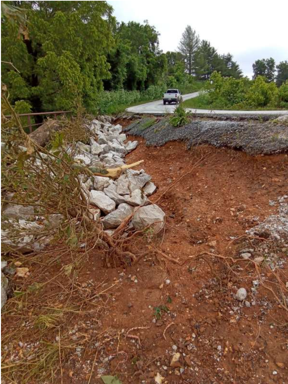
Emergency Procurement #2025-2 Road Damage Picture 2
