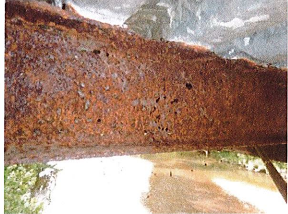
Span 4, Panel 7, Stringer No. 6: 80% section loss to web, 3/16" flange thickness remaining
