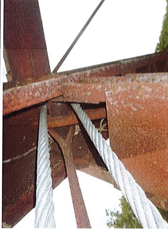
PHOTO 22 SPAN 4, EAST TRUSS, L2-U3: Wire rope sister member added
