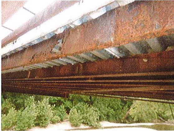
Span 4, Panel 3, Stringer No. 1: 100% section loss to web, serious section loss to flanges
