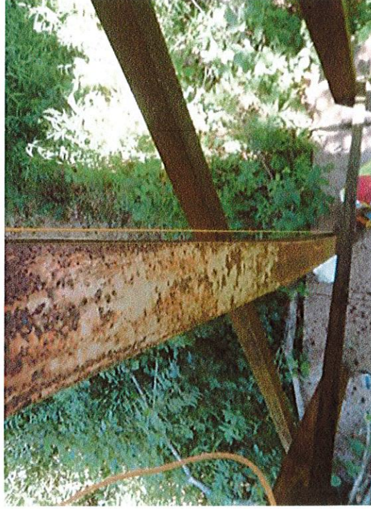
PHOTO 15 BENT 3, PILE 3: Pile is bent 1 1/8" out of plane
