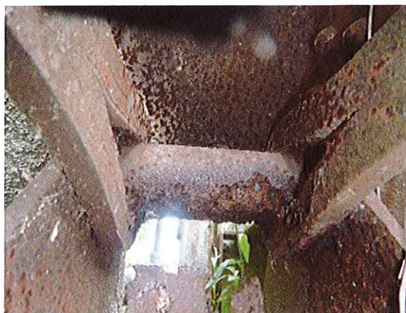
Thru Truss, West Truss, L0: Pin has 3/16" deep pitting on 1/4 of the pin circumference for 2/3 pin length
