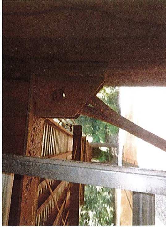
PHOTO 19 BENT 4: Missing pin at top of bent X bracing
