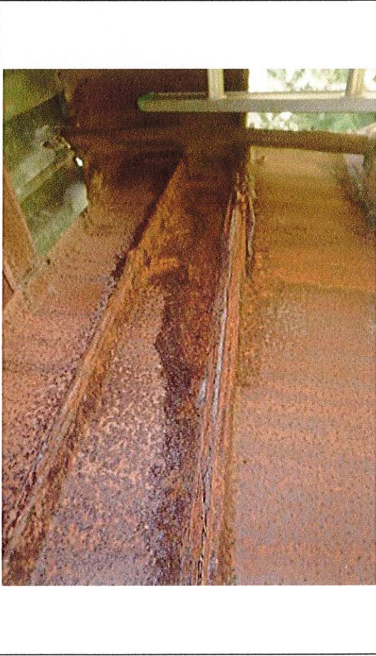
PHOTO 11 SPAN 2, FLOOR BEAM 2: Center member (spacer member) has large corrosion hole at west end
