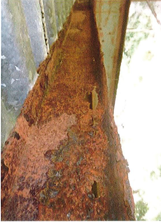
PHOTO 13 SPAN 2, STRINGER 4: 80% section loss to web and bottom flange
