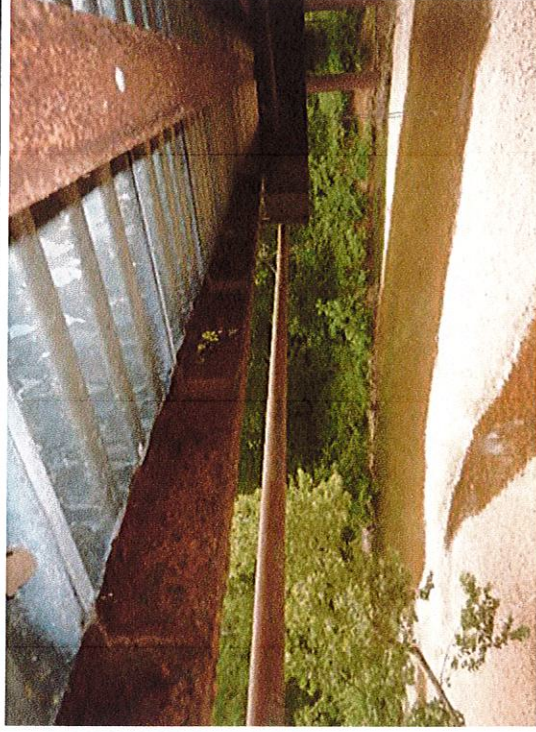
PHOTO 28 SPAN 4, PANEL 1, STRINGER 1: Severe corrosion and section loss in stringer
