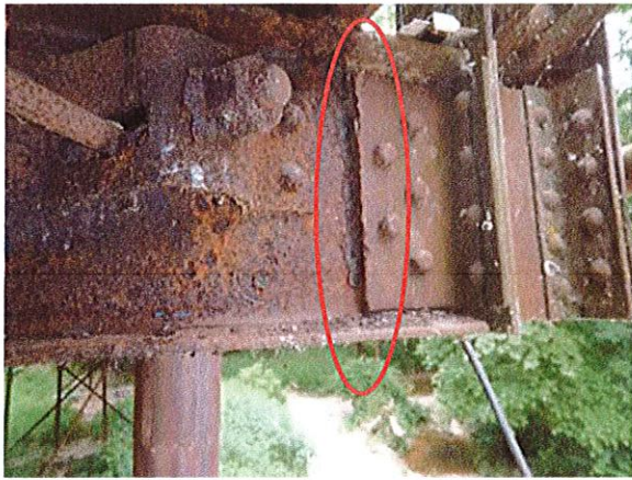
Floor Beam 1, East End, North Face: Serious section loss in web next to connection plate
