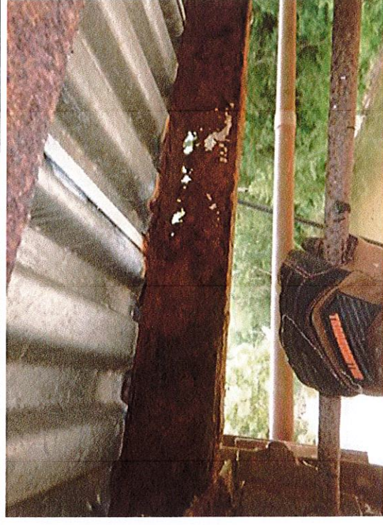
PHOTO 36 SPAN 4, PANEL 4, STRINGER 1: Severe section loss in stringer
