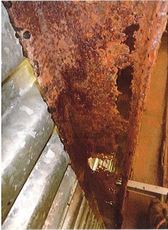
PHOTO 17 SPAN 3, PANEL 1, STRINGER 4: 80% section loss to member
