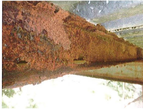
Span 2, Panels 3 and 4, Stringer No. 4: 80% section loss to web and bottom flange
