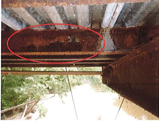
Span 4, Panel 3, Stringer No. 4: Web rusted out near south end
