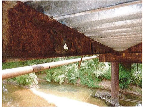
Span 4, Panel 5, Stringer No. 1: heavy pack rust and serious section loss to stringer
