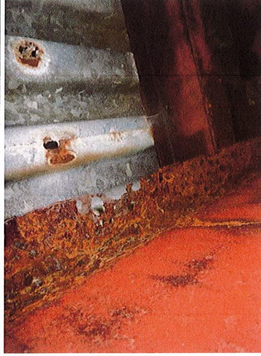
PHOTO 46 SPAN 6, FLOOR BEAM 3: 50%-75% section loss to top flange about 30" from West Girder
