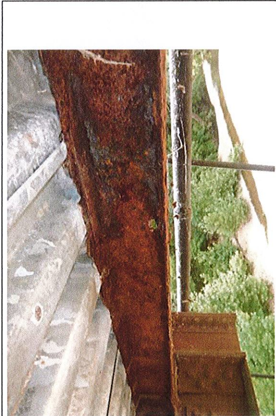
PHOTO 37 SPAN 4, PANEL 4, STRINGER 9: Severe section loss in stringer
