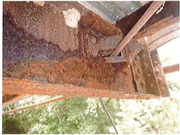
Floor Beam 3, East End: 40% section loss to bottom flange
