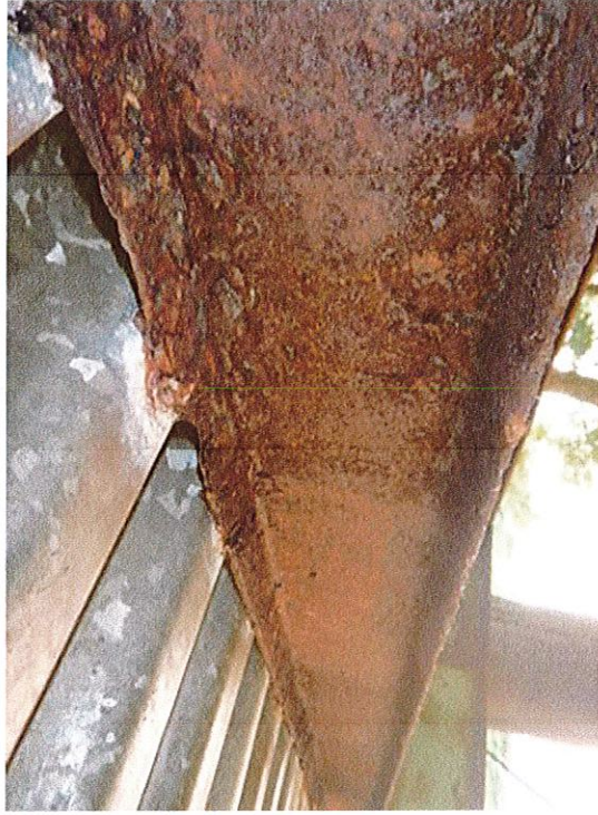
PHOTO 18 SPAN 3, PANELS 3 & 4, STRINGER 5: 50% section loss in member
